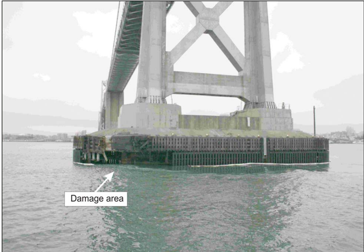
Figure 5. Damaged fendering system at the base of the Bay Bridge Delta tower.
